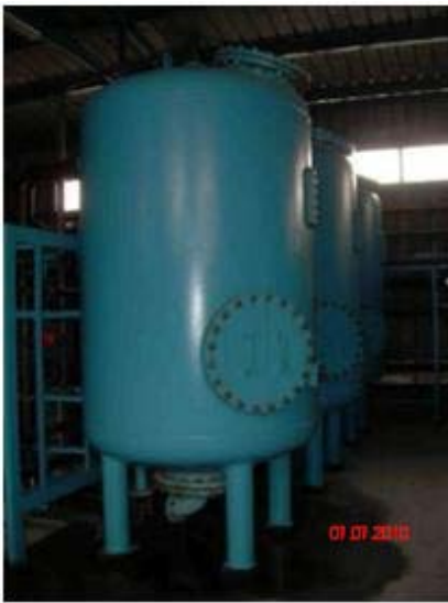
Dual Media Filtration, Sea Water Desalination Plant, Deir Al Balah governorate
