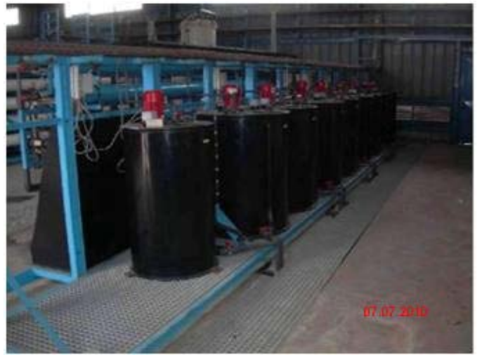
Chemical dosing pumps, Sea Water Desalination Plant, Deir Al Balah governorate
